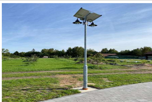
Anwohnerstraße Aivis-Mertens in Lättland Small road lighting Aivis-Metrens in Latvia
